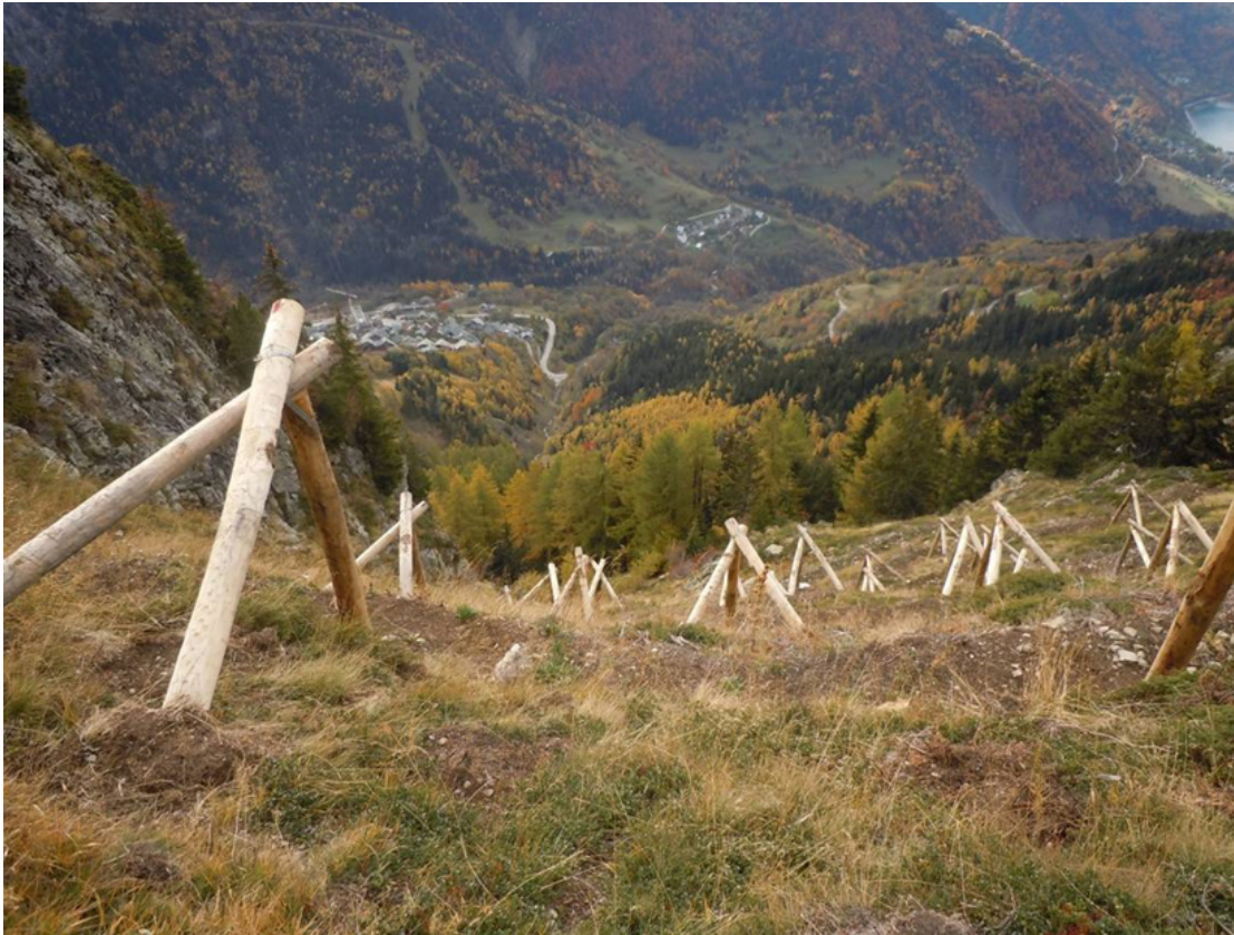
Figure 21. Real world mitigation measure at Capet forest
