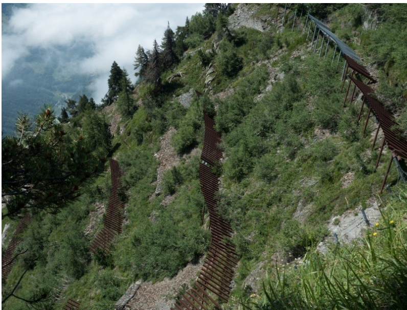
Figure 14 Soil stabilization in the Thiel corridor, as proved by the presence of dense 25-year-old groups of aspens, silver birches and mountain ashes below the snow rakes
