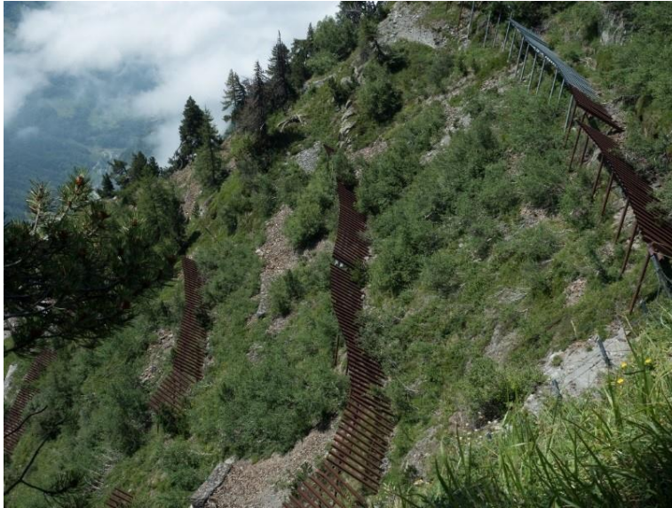
Figure 10. Soil stabilization in the Thiel corridor, as proved by the presence of dense 25-year-old groups of aspens, silver birches and mountain ashes below the snow rakes.
